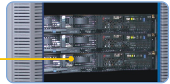
IBM Server Application
